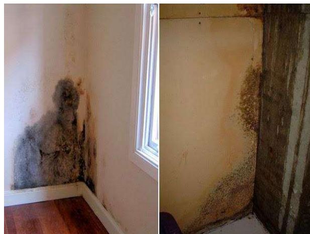
Major Damage caused by Slow leak in Water Heater
